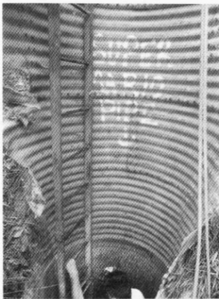
Our entry to the wet side of the site via the remains of an emergency escape shaft
